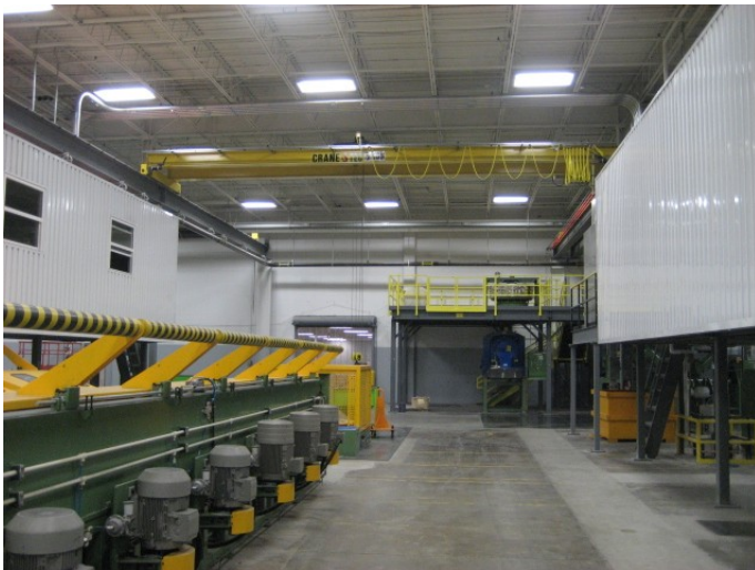
5 ton double girder crane and runway system
