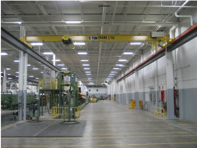
5 ton crane and runway system
